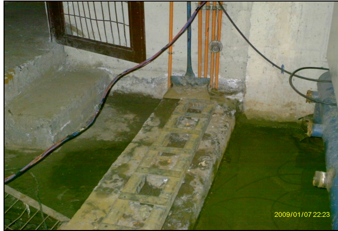
MANIFOLD SIN BOMBAS
