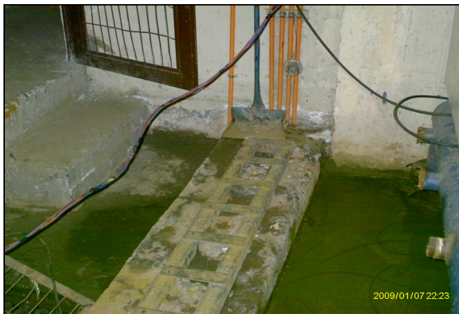
MANIFOLD SIN BOMBAS
